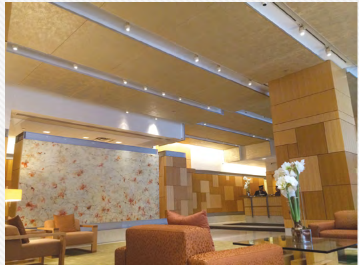
New LED lighting in the lobby of The Cielo.
